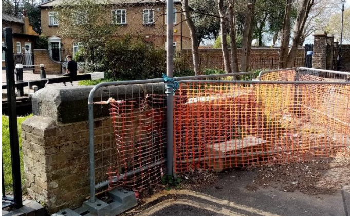
Parnell Rd. Bridge left unrepaired in 2020 .
